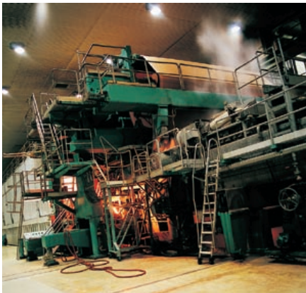
Figure 5: VST-SE for paper making using low pressure steam for paper making
