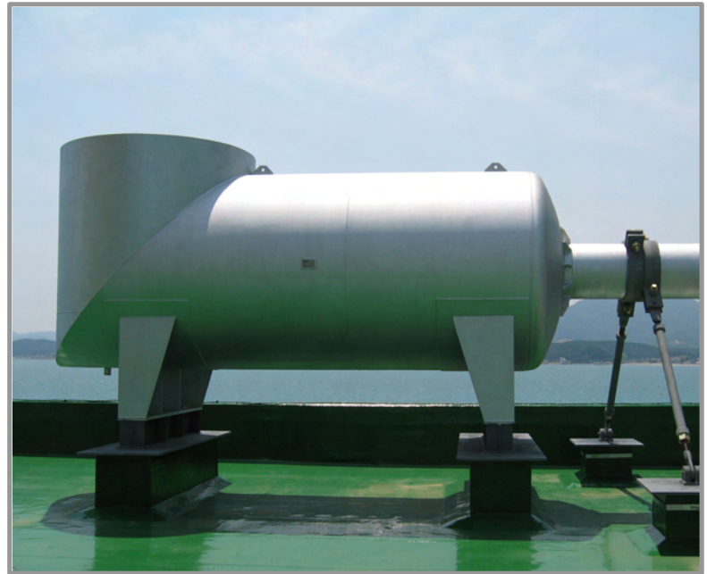
The newly installed silencers reduce noise to 74dba
